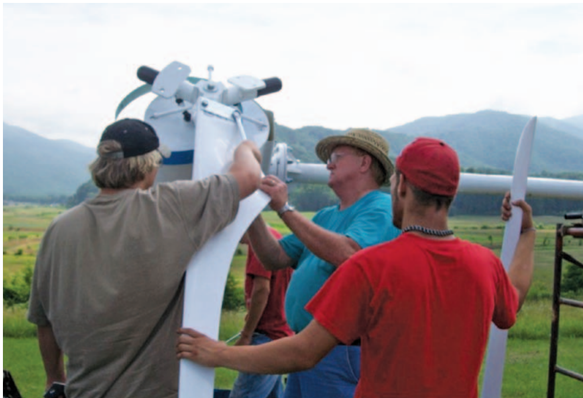
Ronnie Trout worked with students to connect a Kestrel 3-kW machine to the 119' guyed tower that was designed and constructed at Morgan County Career and Technology Center. Photo courtesy of Brandon Blevins.
