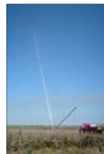
Installation of 50-m Met tower by AEI of West Texas A&M at GSA Border Station site in Donna, TX.
