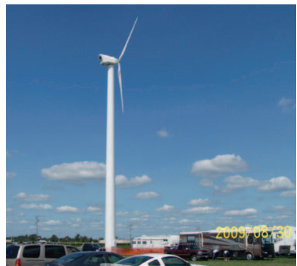
A 100-kW Northwind 100 turbine installed at the Farm Progress show site generated a lot of interest and drew attendees to the WPA exhibit for more wind energy information. Photo credit: Dan McGuire.
