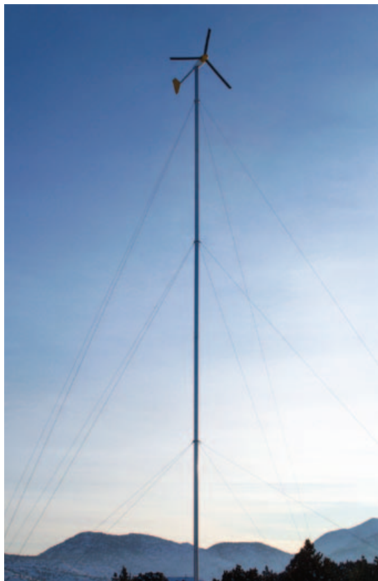
Joe Pizur installed a Bergey XL-1 turbine on a 60-foot tower at his residence in the Virginia City Highlands, Nevada. Mark Harris/PIX16742.
