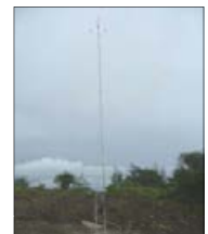
60-m Met tower installation at Naval Magazine on ridgeline in western Guam. Installation by DNV-GE.
