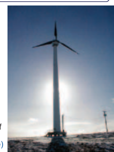
Three Northern Power Systems Northwind 100/19 (100-kW) on special permafrost foundations.
