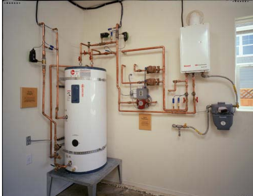
Figure 13. ST system plumbing
