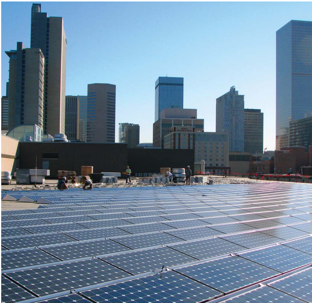
Namaste Solar was responsible for this 300 kw PV rooftop installation on top of the Colorado Convention Center in Denver, Colorado. (Namaste Solar Electric/PIX18044)
