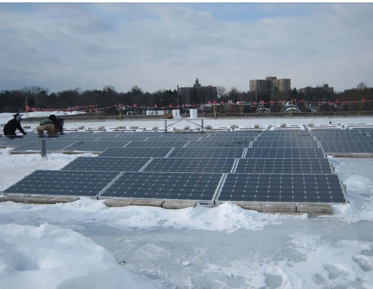
Nearly 2,000 solar panels installed at the Veterans' Affairs Regional office and Insurance Center in Philadelphia produce over half a million kilowatt-hours of solar electricity annually. (The U.S. General Services Administration/PIX18066)
