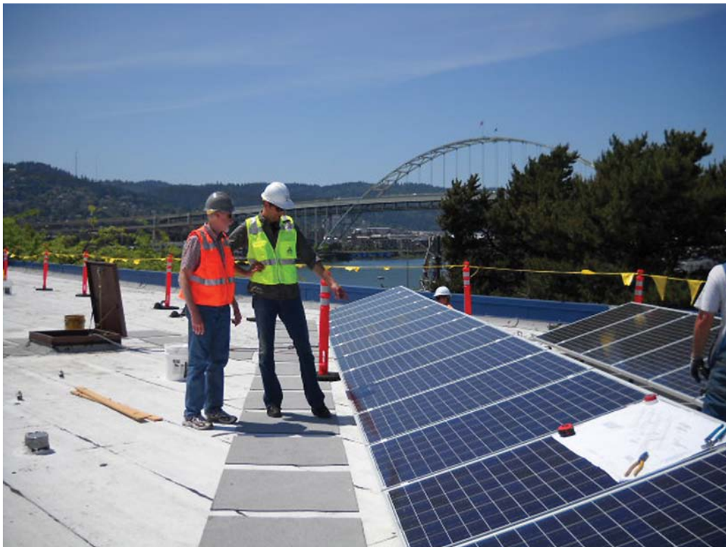
This 12 kW PV array is the largest system entirely owned by the City of Portland. (City of Portland/PIX18048)
