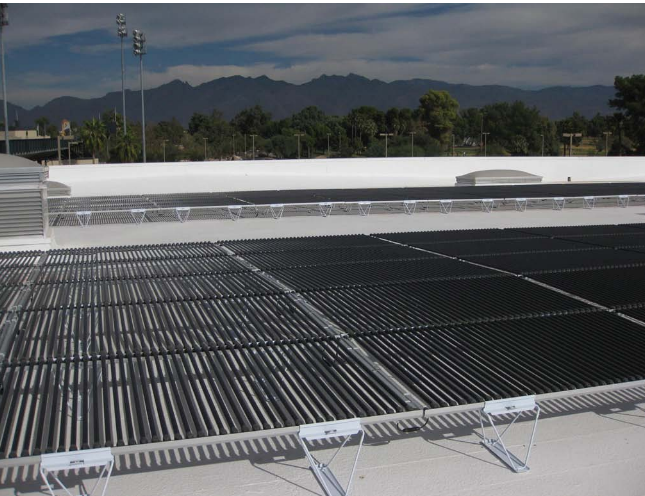
Cylindrical Solyndra PV panels are installed on top of the City Parks Warehouse in Tucson, Arizona. (City of Tucson /PIX18041)
