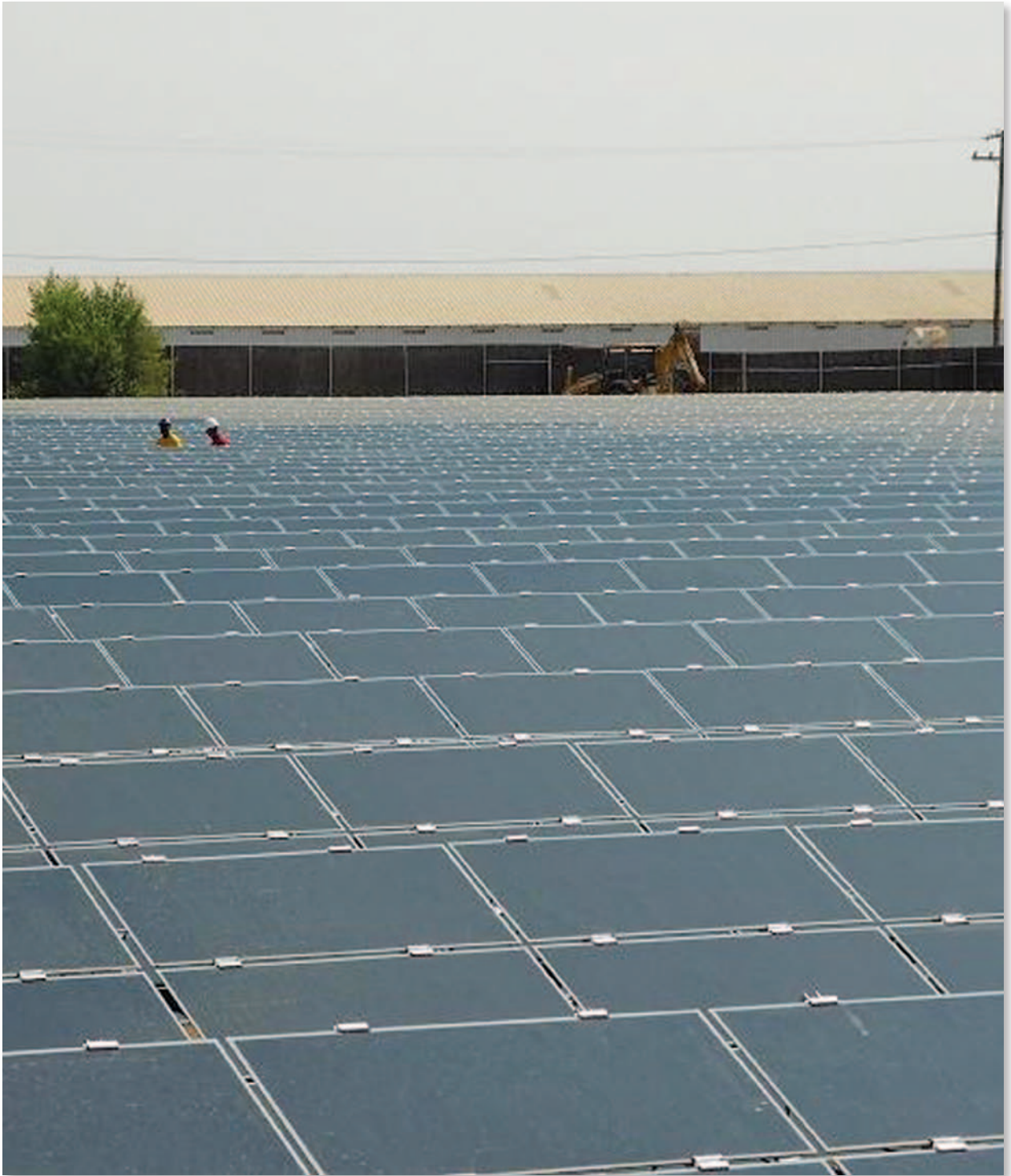
SMUD's SolarShares Installation
