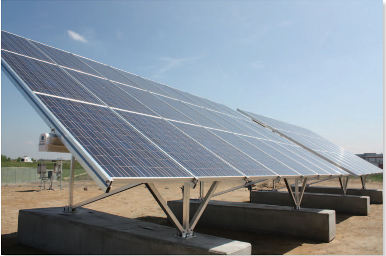
United Power's Sol Partners Installation, Colorado
