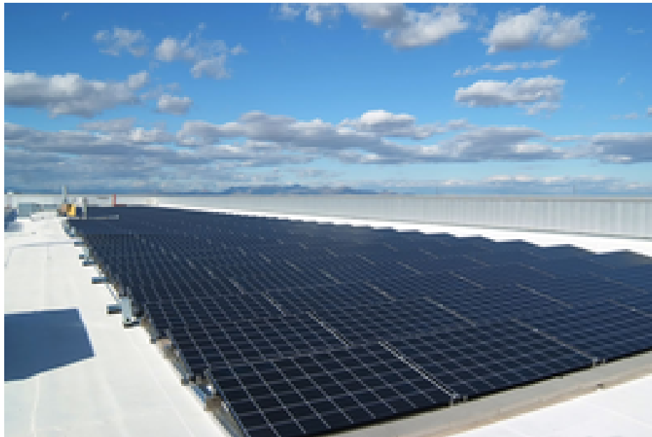
Figure 20.0: Rooftop photovoltaic array
