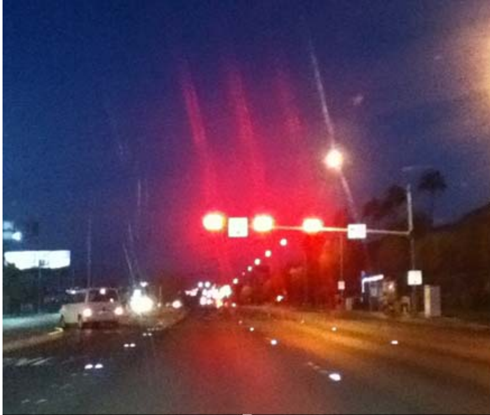
Figure 3-13. View of Activated PHB System at Night
