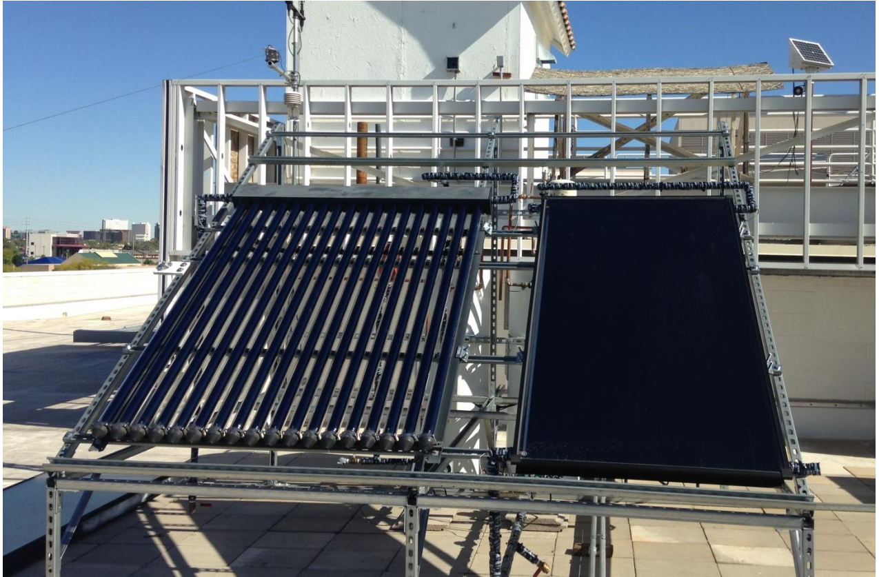
Figure 8: Picture of System Looking North
