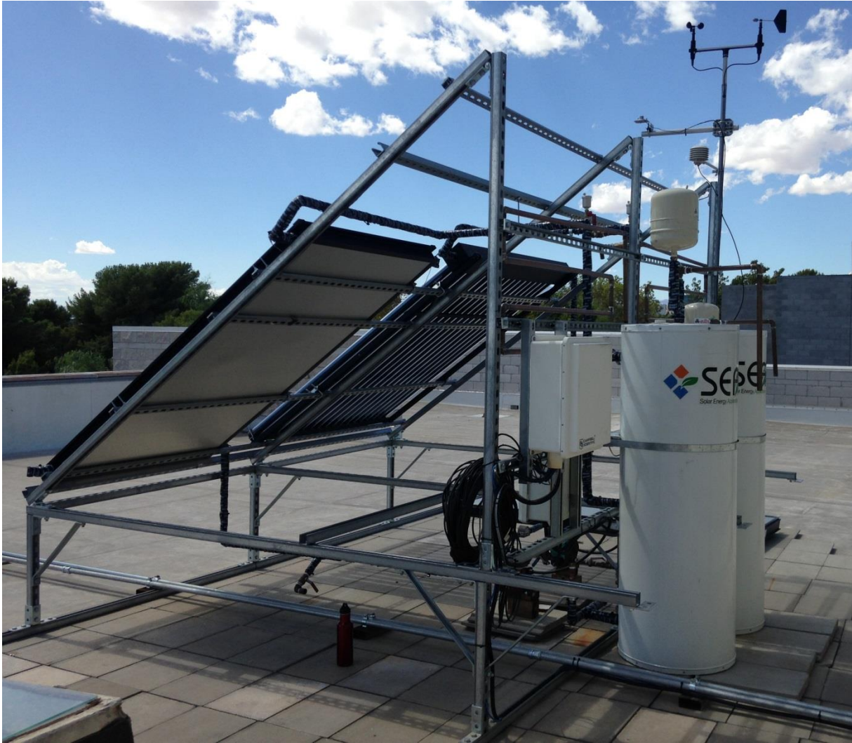
Figure 10: Picture of System Looking Southwest
