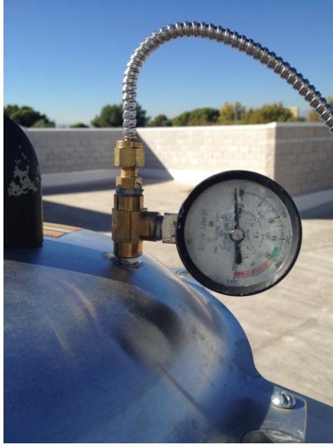
Figure 21: Piping where the thermocouple and pressure gauge connect to the lid
