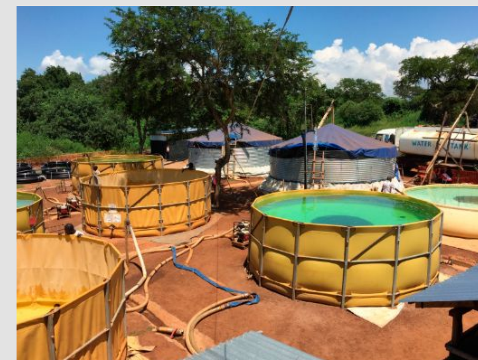
Fig. 4 - Emergency Chlorination Tanks 2
