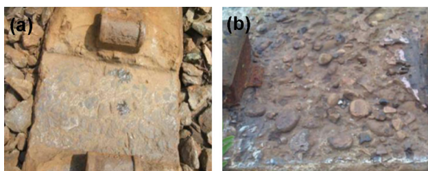
Fig. 1 Prestressed concrete rail-seat abrasion: a Reiff et al. [13], b Zeman et al. [7]
