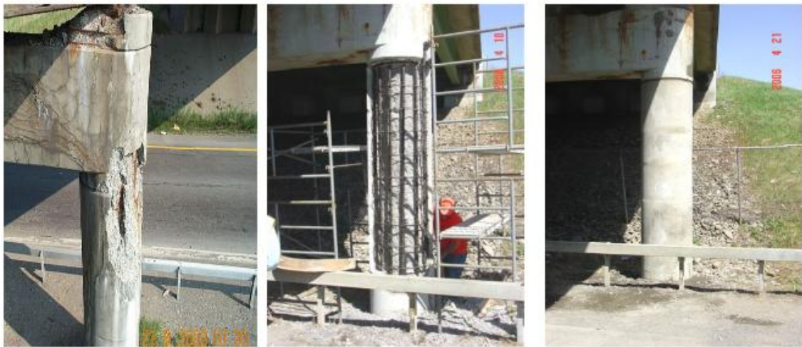
Figure 10. (Left) Corrosion Damage, (Center) Removal of Concrete and Repair Reinforcement, and (Right) Replace Concrete (NYDOT, 2008)
