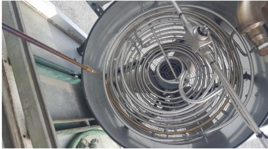
Figure 14. Air Cooled Heat Rejection Heat Exchanger
