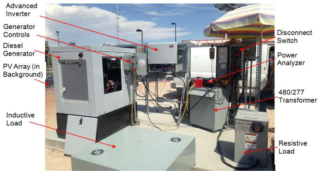
Figure 4.5 An Image of the Advanced Inverters Experimental Test Setup.
