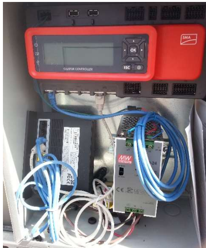
Figure 2.4 Image of Inverter Controller with Router.
